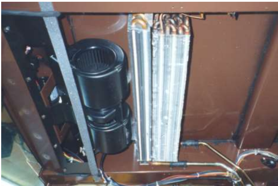
Evaporator in place beside heater coil.
