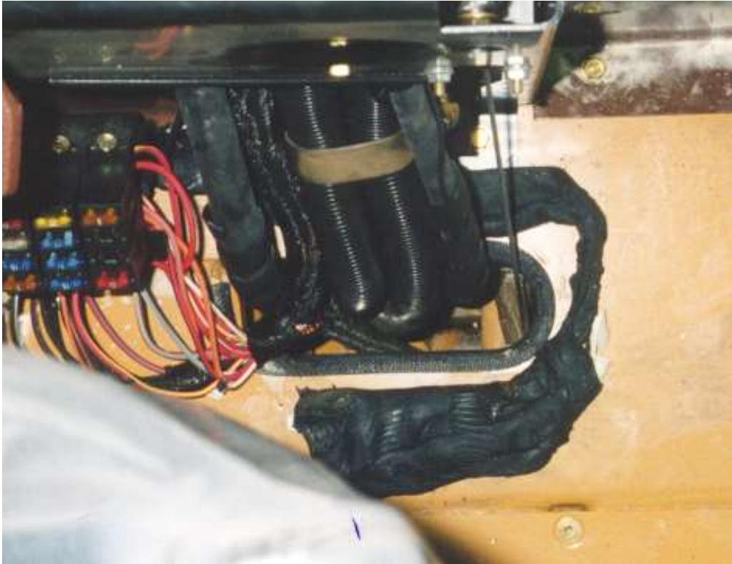
Hoses routed through floor of cab.
